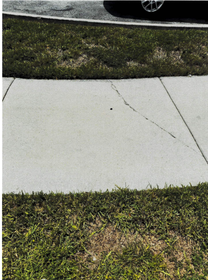
Sidewalk Slab Replacement (although not a trip hazard, we want to replace it since we are performing concrete work)
